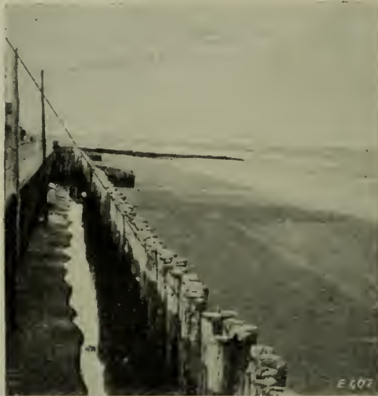
FIG. 3. SHOWING SCOUR BEHIND SHEET PILING.
